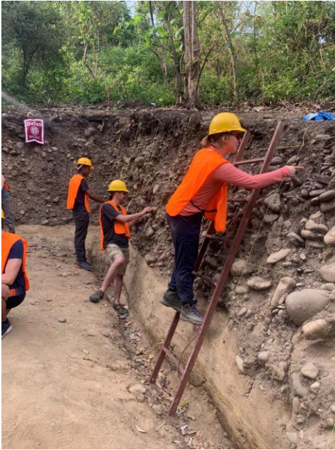
Students cleaning the walls of a trench near Ramnagar India, for Shreya Arora's short term titled "Investigating Past Earthquakes in the Western Himalayas" (May 2023).
